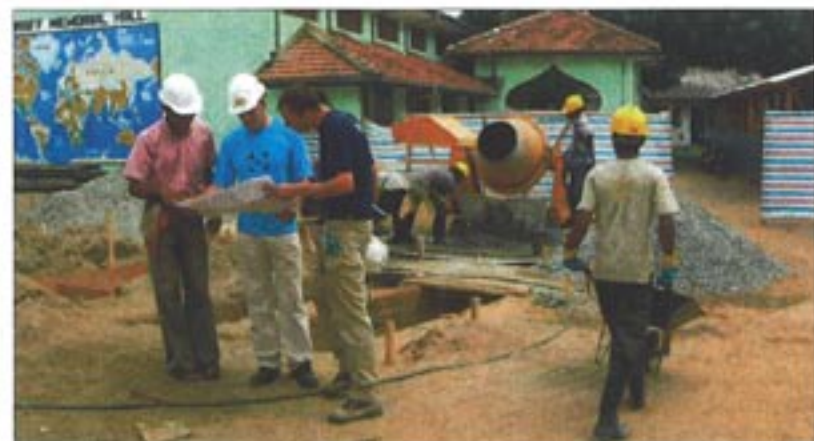
GOAL Schools Project Manager Mark Ford and GOAL Project Engineer Stephen McElheney reviewing details with a contractor, Sri Lanka
