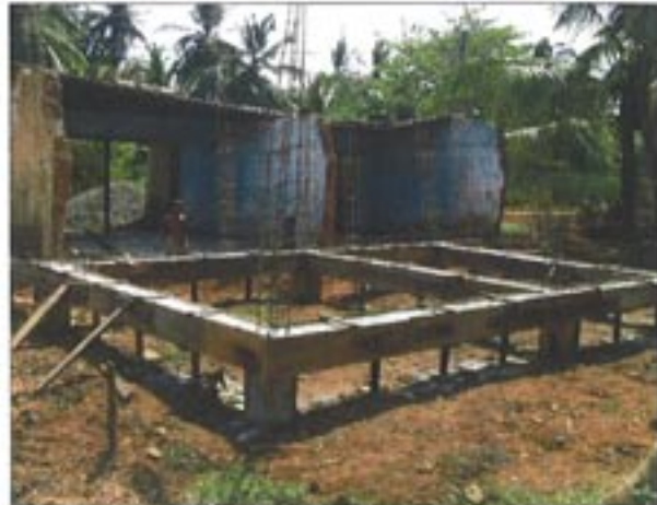
A new house being built on the original site of a destroyed house in Sri Lanka.
